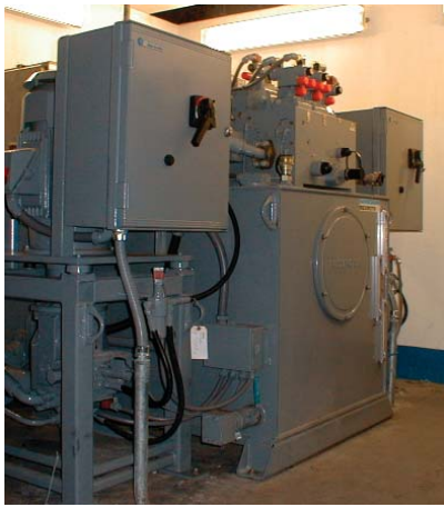
Bosch Rexroth hydraulic power units operate the miter gate cylinders. Each cylinder is operated by one power unit.
