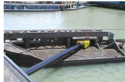
The hydraulic cylinder is attached to the miter gate. Bosch Rexroth’s black Ceramax piston rod coating helps protect against corrosion.
