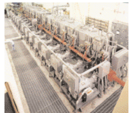
Central Hydraulic Systems
